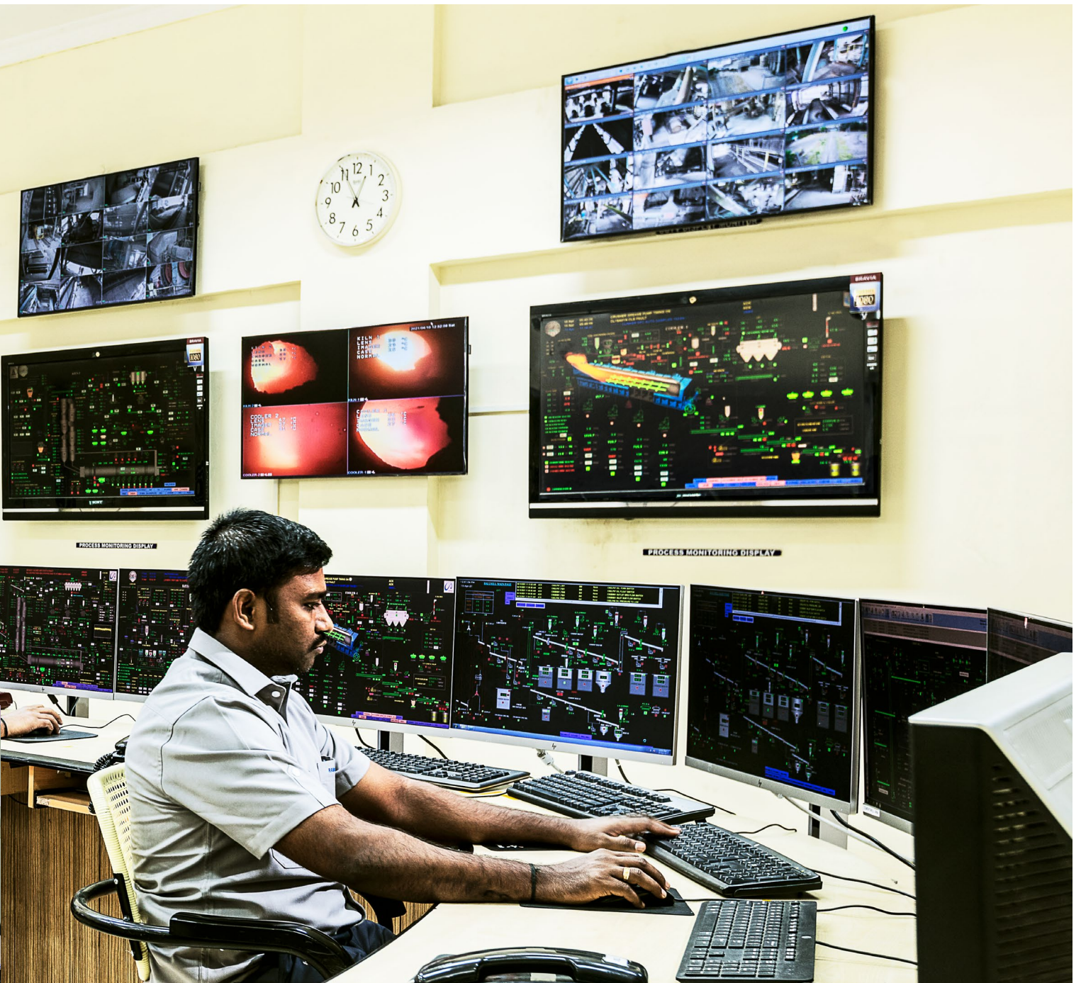
A Central Control Room monitoring the plant operations
